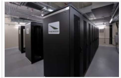
Pinewood Data Centre
